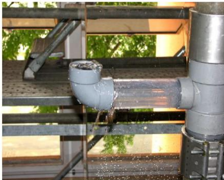
Photo 1: Spouting of water from backflow pipe
