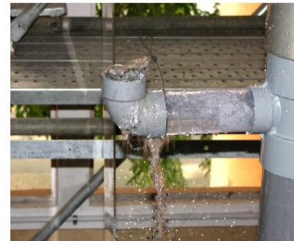
Photo 2: Spouting of water from backflow pipe
