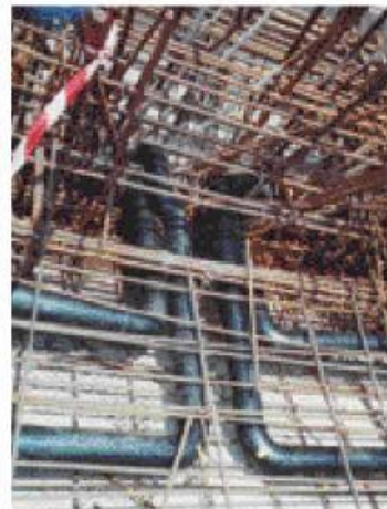
Horizontally laid pipes casted within concrete structure of the sloping gutter system. Specific installation procedure is carried out to ensure that during concrete casting, it does not affect the integrity of the pipe walls.
